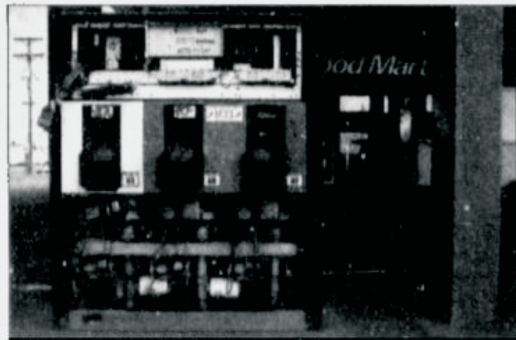
A gas pump stripped of cover, pumps and power stands Tuesday at the closed Chevron on the corner of Pines and Sprague in Spokane Valley.
